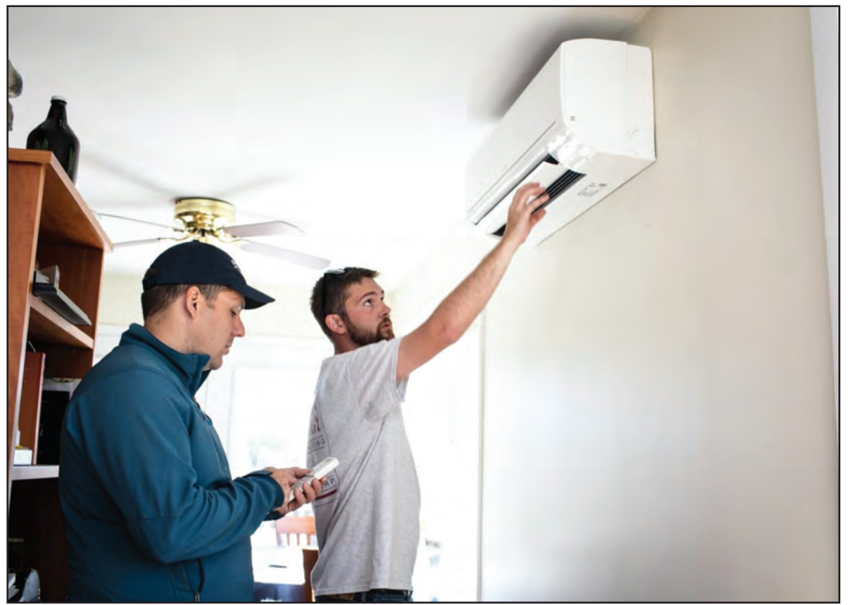
CODY STEPHENSON, A contractor with Vermont Energy, installs a heat pump in a Vermont home a few years back. Photo courtesy of Efficiency Vermont
