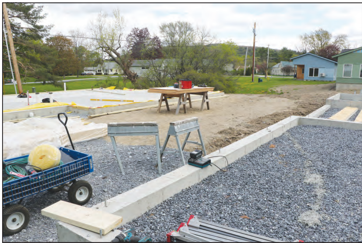
MOST OF THE construction volunteers for Habitat for Humanity of Addison County are knowledgeable about building basics, so this Gorham Lane worksite will seem familiar to them. Independent photo/Steve James
