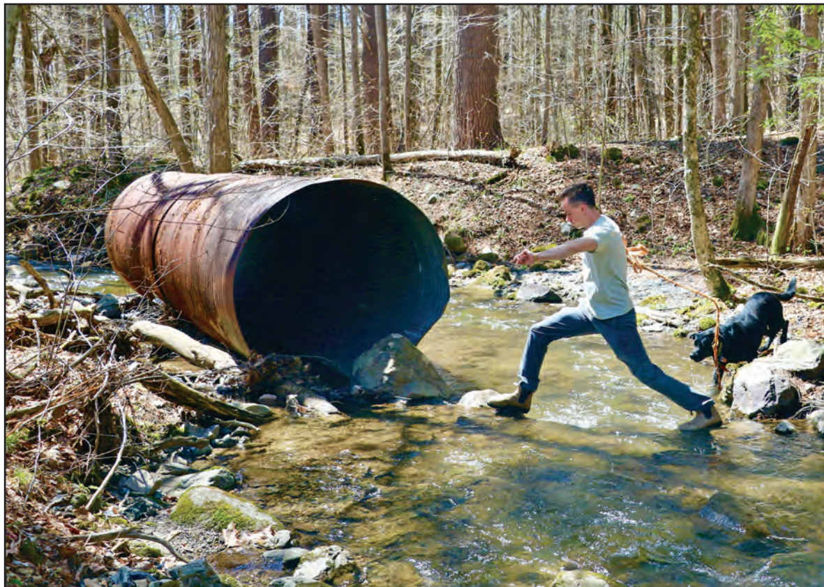
SAM PEISCH, MONKTON selectboard chair, and his dog, Lupin, traverse a stream near Piney Woods Road. It was significantly damaged in a July 2024 storm, which carried this culvert around 25 yards from its previous spot to where it now sits in the stream.
