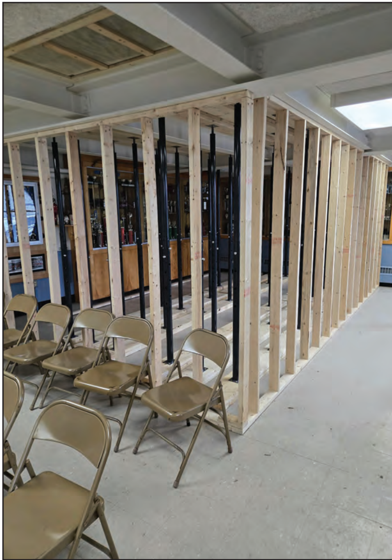
LALLY COLUMNS hold up the ceiling in the basement of the Vergennes Fire Station as a temporary fix. A recommendation committee began meeting in February to think through how to address this, and other issues with the building.
