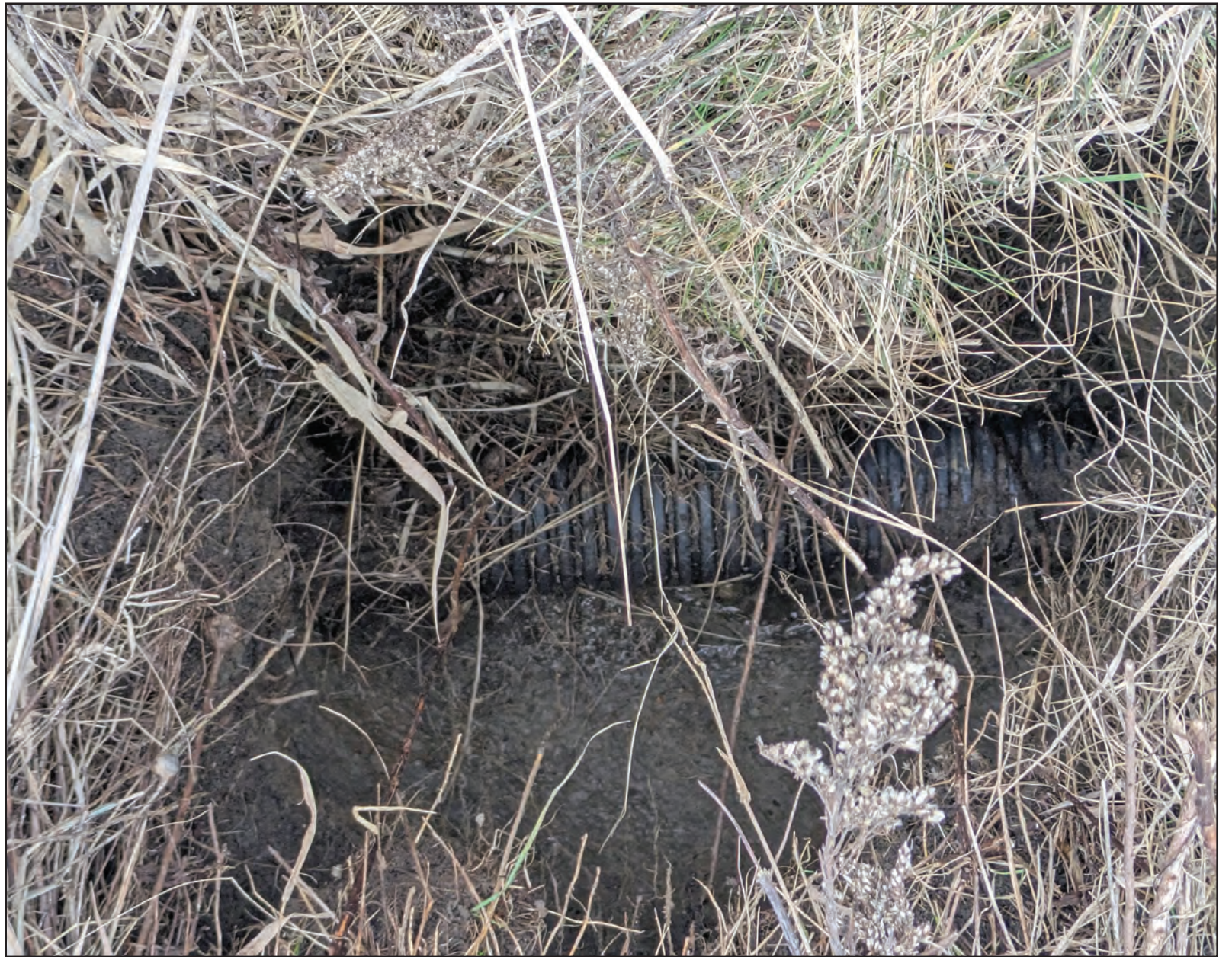
MONKTON RESIDENT Nate Palmer found this sink hole near his property off Rotax Road. It has exposed agricultural drainage conduit, and Palmer is concerned Vermont Gas System’s natural gas pipeline might be shifting and spurring more sinkholes that could affect farming and public safety.
