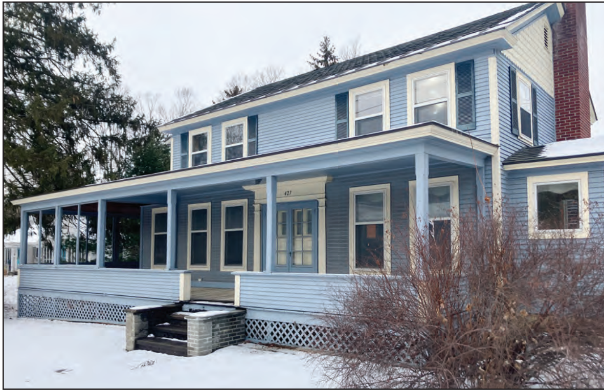
THIS HOME AT 427 East Main St. in East Middlebury is being renovated so that Addison County Home Health & Hospice can run it as a new care home for folks with chronic ailments who can no longer live independently.
