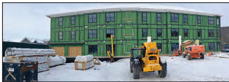
A 35-UNIT RENTAL property takes shape in the heart of the Stonecrop Meadows subdivision, rising above land off Middlebury's Seminary Street Extension.
