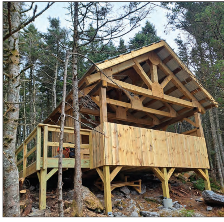
THIS NEW SHELTER under construction at the Battell overnight site on Mount Abraham will be featured in the Bread Loaf Section annual meeting on Sunday.
