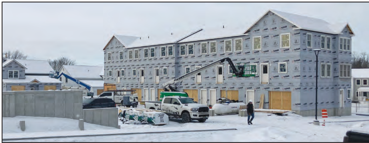
WORKERS AT MIDDLEBURY'S Stonecrop Meadows subdivision do exterior and interior labor on duplexes (left) and a multi-unit standalone building (right). Six units off Seminary Street Extension are already occupied and 70 could be ready for habitation by year's end.
