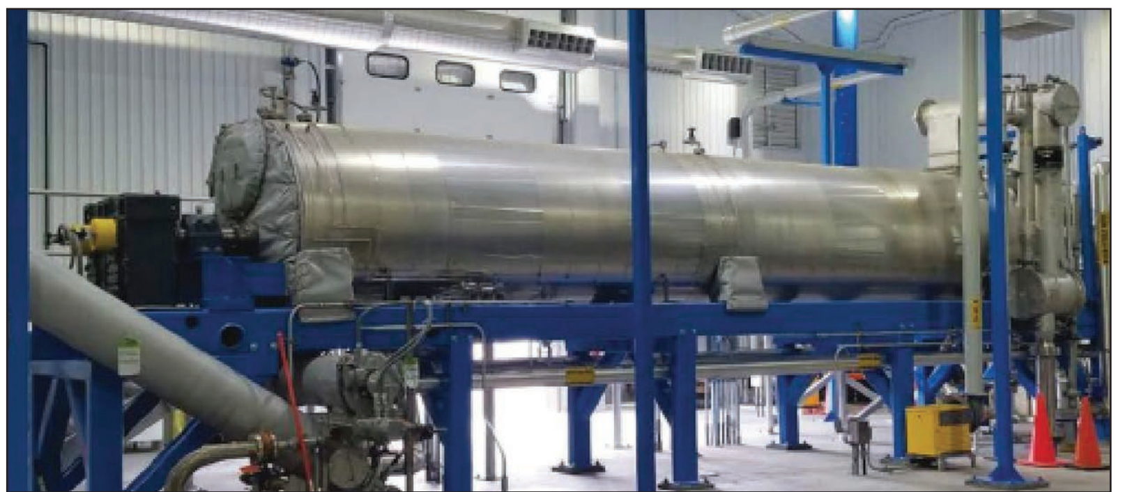
THIS BIOSOLIDS DRYER is being advanced as part of a series of major upgrades at the Middlebury wastewater treatment plant. Photo courtesy of Wright-Pierce
