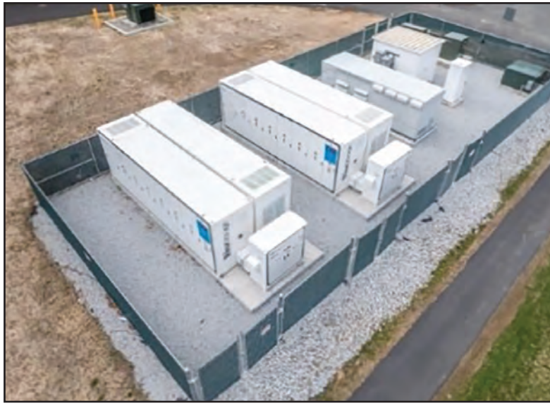
THIS LIGHTSHIFT BATTERY storage plant in Groton, Mass., is similar in appearance and scale to the one proposed for a Pantone Road lot in Vergennes. The facility could store 5 megawatts, enough to power more than 4,000 homes.
