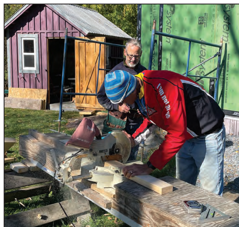
HOMES FIRST, A nonprofit working to solve the housing shortage, is building a roughly 527-square-foot home, which will be rented at a long-term, affordable rate — as will an adjacent two-story home.
