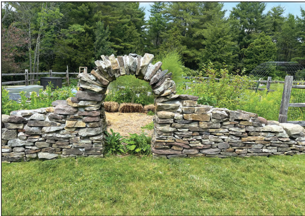
Stone mason Jamie Masefield created this entrance arch at the Monkton Central School vegetable garden
