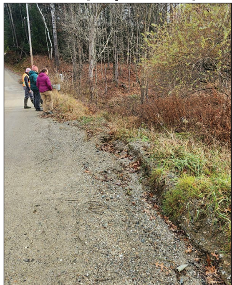
LEWIS CREEK ASSOCIATION'S Kate Kelly and SLR Engineers look at Lewis Creek with visible road erosion at the Common Ground Center. This erosion will be addressed by a drainage improvement project funded in part by a grant from the Vermont's Clean Water fund.
