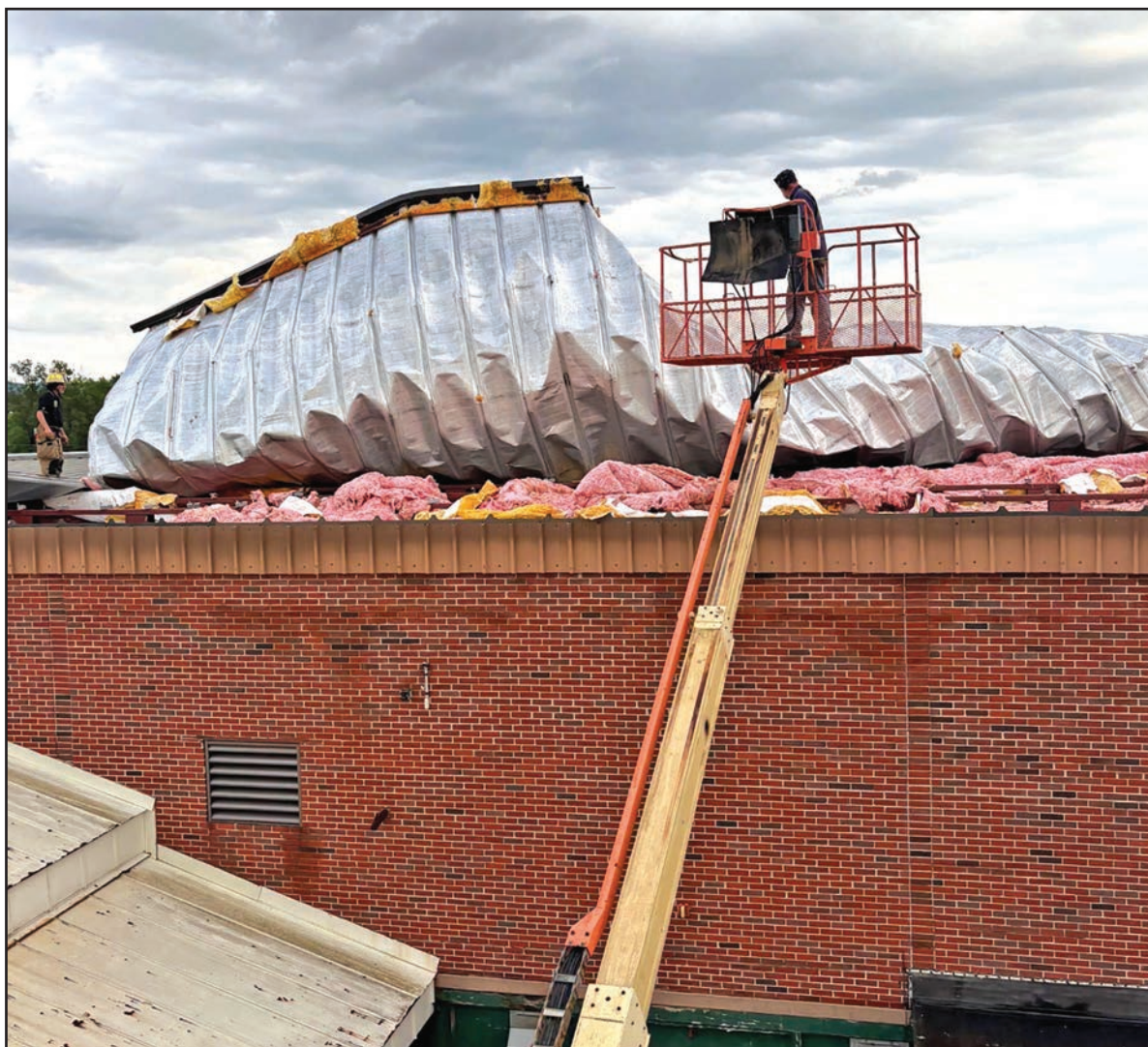
VERGENNES FIREFIGHTERS USING the department's tower truck responded to Middlebury Union High School this past Thursday evening to help secure a portion of the roof that was blown off by high winds.
