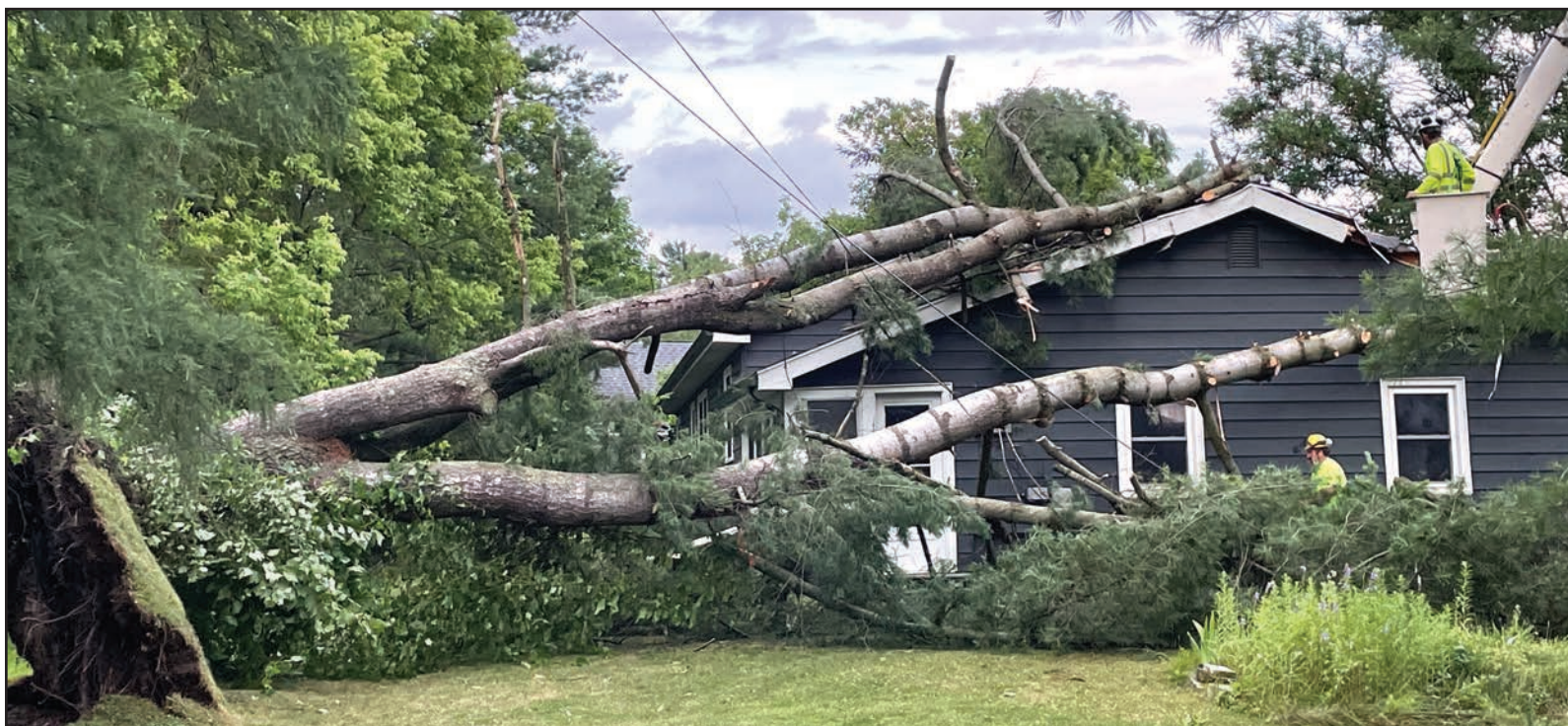
TREES FELL ONTO this Danyow Road home in Middlebury during the July 10 storm; no one was injured. There were other homes in the area that also saw damage.
