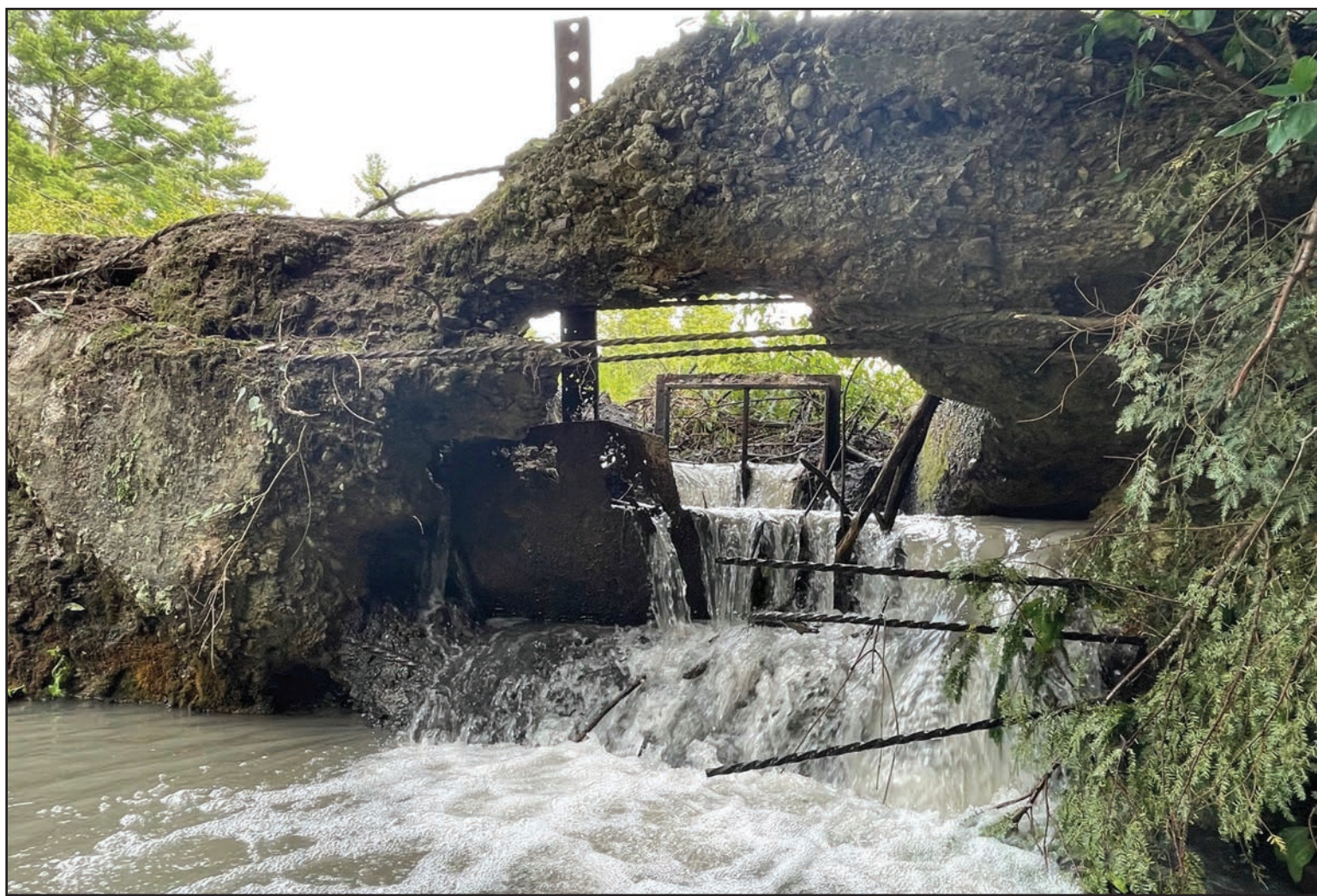
THE OLD WAINWRIGHT Mill Dam has been removed from its Salisbury location, allowing Tributary 10 of the Otter Creek to pass freely through its channel for the first time in 219 years.
