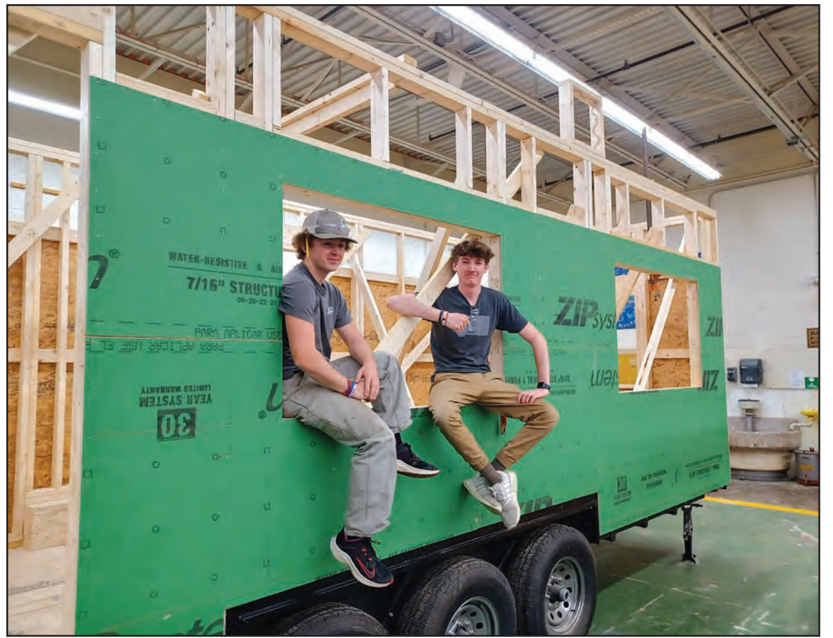
HANNAFORD CAREER CENTER students who learned practical carpentry skills proudly show off the tiny house they were helping build.
