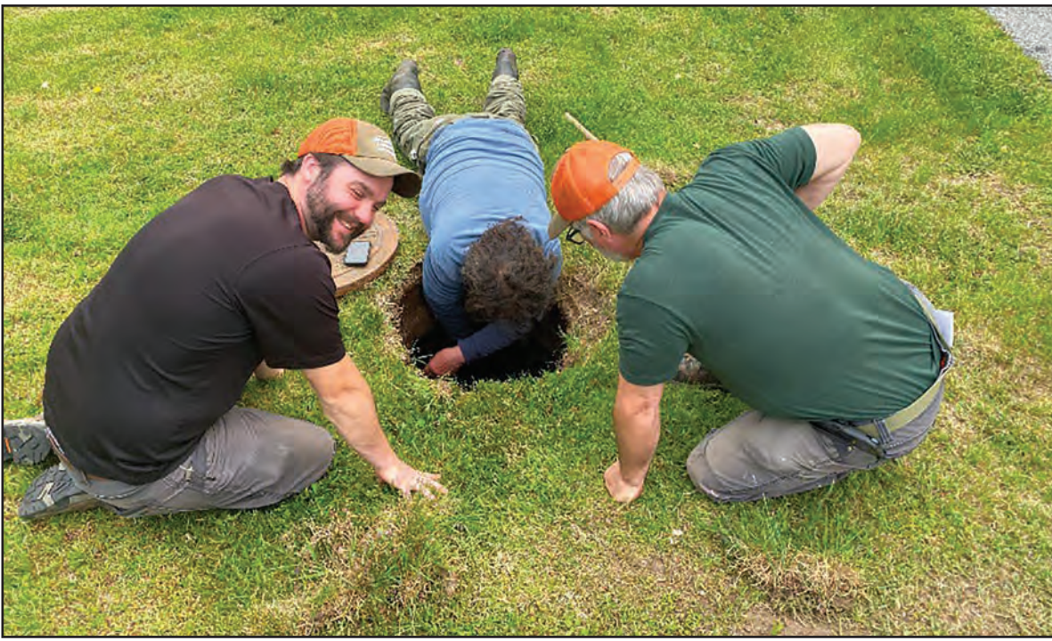
BEN KIVLEN (LEFT), Donnie Wall (right) and a tech from J&A Pump investigate a malfunctioning sewer pump at Weybridge Street Apartments.
