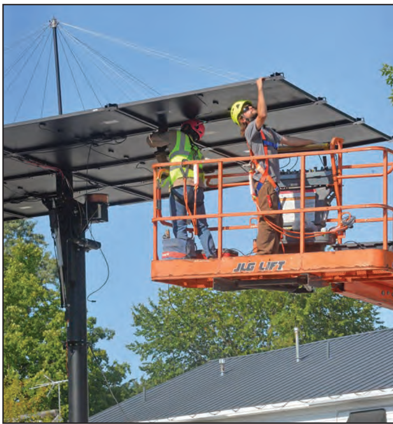
INSTALLERS SET UP a Solaflect Energy solar electric vehicle charger next to the Marble Works parking lot in Middlebury last month. In Middlebury, the Norwich company set up two stand-alone EV chargers powered only by renewable solar energy.
