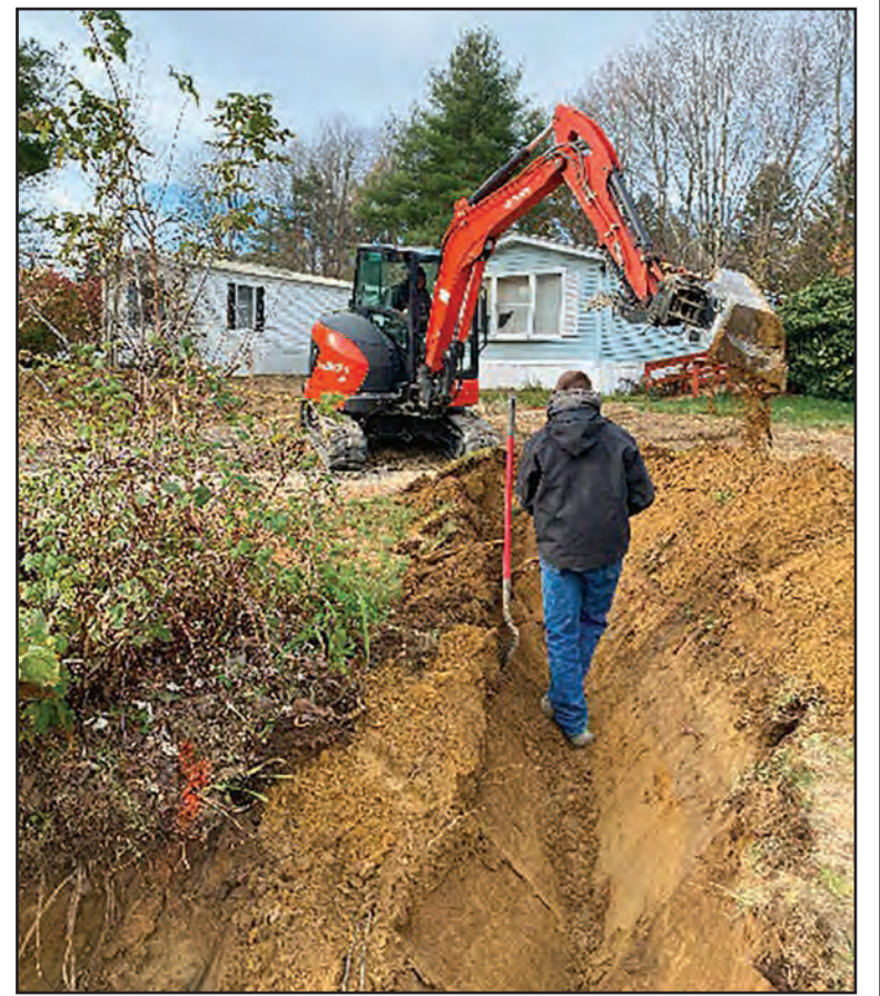
A CONTRACTOR LOOKS for the source of an electrical problem in Lindale Manufactured Housing Community in Middlebury.
