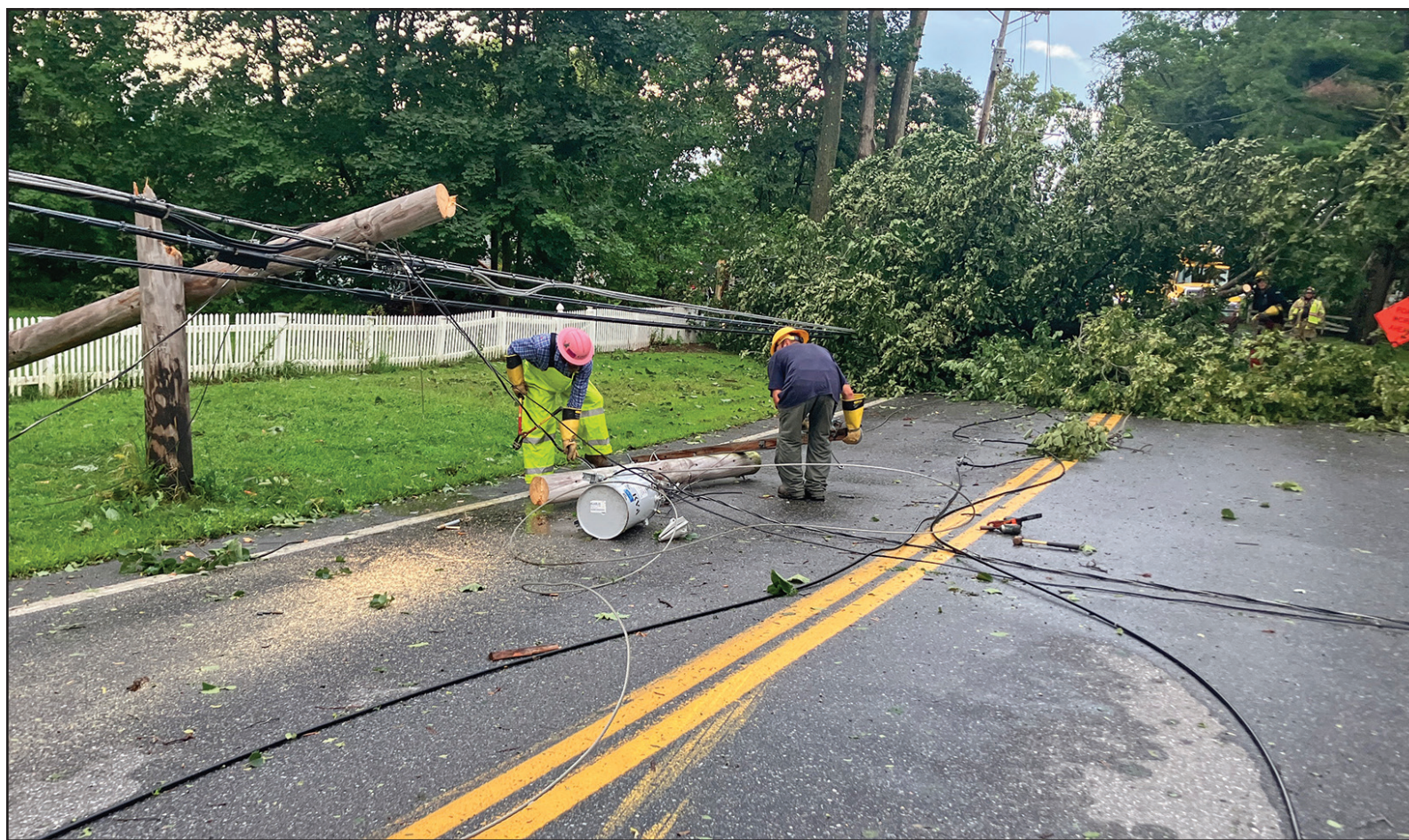
GREEN MOUNTAIN POWER linemen pick up an electricity transformer that was broken when it smashed onto Route 116 after its utility pole fell during the 60 mph winds on Friday evening. Power was restored in the area by Saturday morning.
