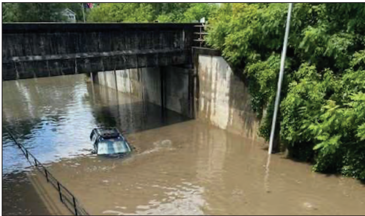
MIDDLEBURY OFFICIALS ARE scoping out potential ways to prevent flooding at the Seymour Street underpass. The underpass has flooded twice during the past year, which has neighbors concerned about emergency responders' ability to access the neighborhood during major rainstorms.
