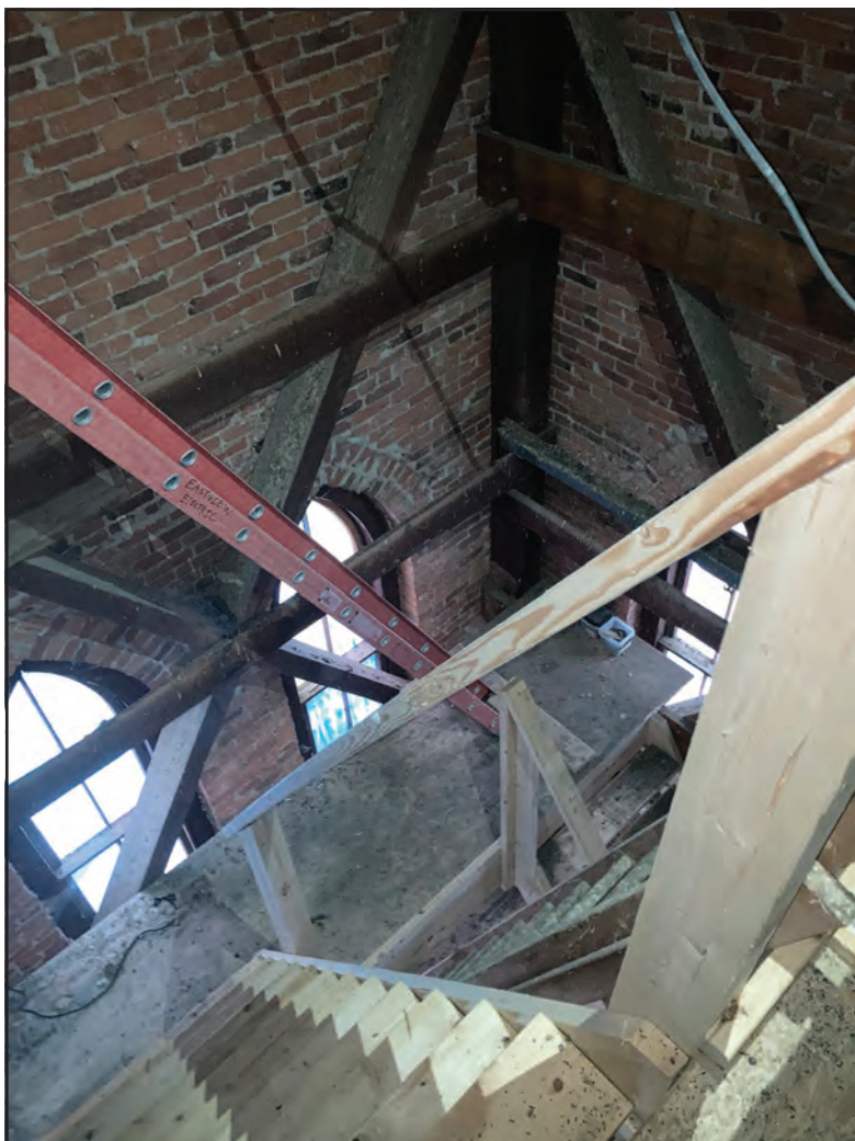
THE BELLS IN St. Peter's Church in Vergennes should ring again this Sunday to celebrate the church's 150th anniversary. Creating safe access to the bells in the belfry atop the 125-foot-tall tower was a challenge. Volunteers cleared pigeon waste, reinforced staging, and replaced rickety, aging extension ladders with new, sturdy ship-style ladders.
