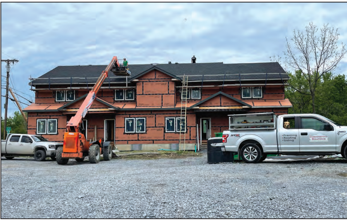
WORK ON A two-building, nine-unit condo/apartment project on Otter Creek in Vergennes began again this month after its developer, city firm Cornerstone Solutions LLC, obtained an Act 250 permit. The company halted work on the so-called "Portage Project" almost a year ago when state officials ruled an Act 250 permit was required. An unsuccessful appeal of that decision further slowed progress on the West Main Street development.
