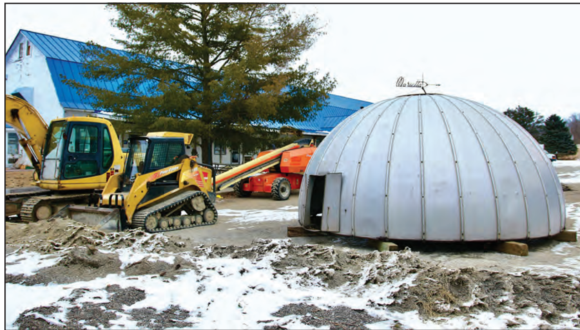
FOLKS FROM NOP’S Metalworks were busy this week dismantling and removing the former 80-foot-tall, 70-year-old silo that was a popular feature of the Bridge School and a local landmark for those entering and exiting Middlebury’s northern gateway. The top will be used in a new gazebo on the same site.
