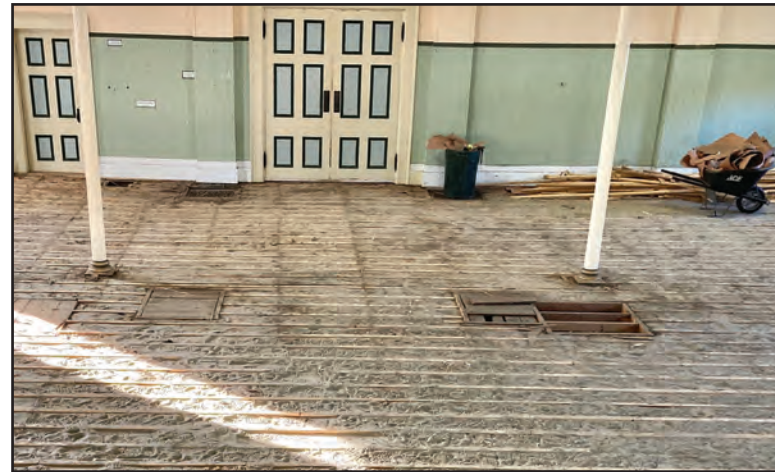
WHEN THE FLOORBOARDS were pulled up, workers found the space between joists was filled with sand — a decidedly low-tech method to muffle sound when the floor of the 160-year-old building was installed. The sand was shoveled out (filling an entire dump truck), and a new subfloor was installed.
