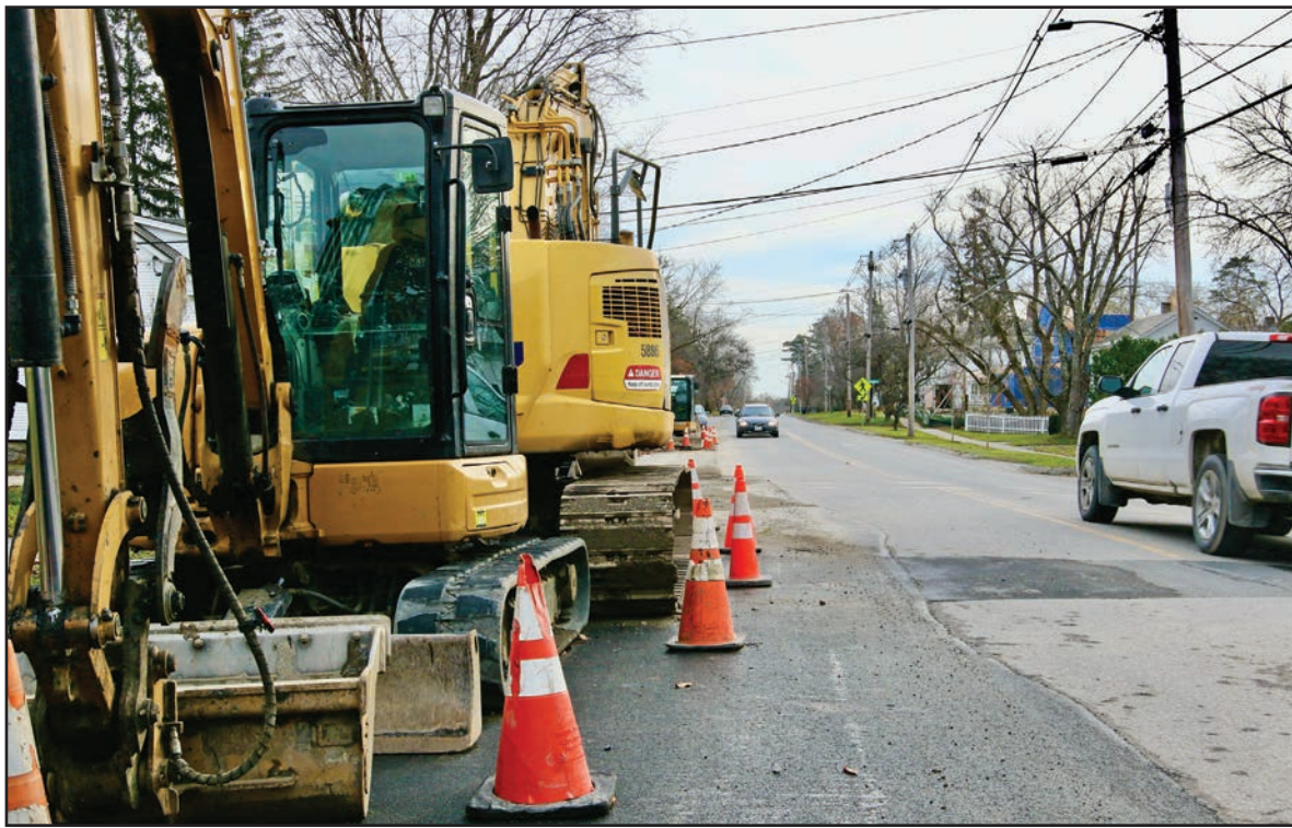
Work on Phase 4 of a sewer and stormwater infrastructure refurbishment project on South Street in Middlebury is underway now. On Town Meeting Day Middlebury voters will decide whether to fund Phase 5 of the project.
